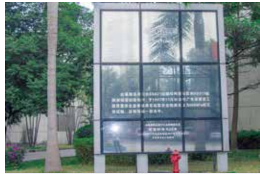
▶ This is a glass curtain wall for sealant durability test which was set up in 1997.
