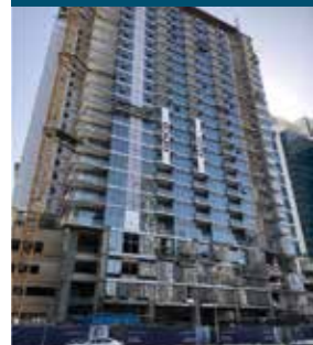
Ginco Resence Tower
